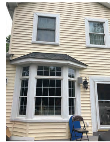
PROPOSED VINYL SIDING TO MATCH THE MAIN HOUSE, BY "PlyGEM" or EQUAL, COLOR: YELLOW
