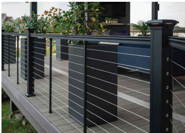
CABLE RAILING w/ BLACK ALUM. POSTS by "KEYLINK"
